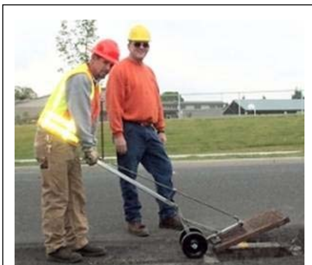
Figure 8: City Operations designed grate lifter
